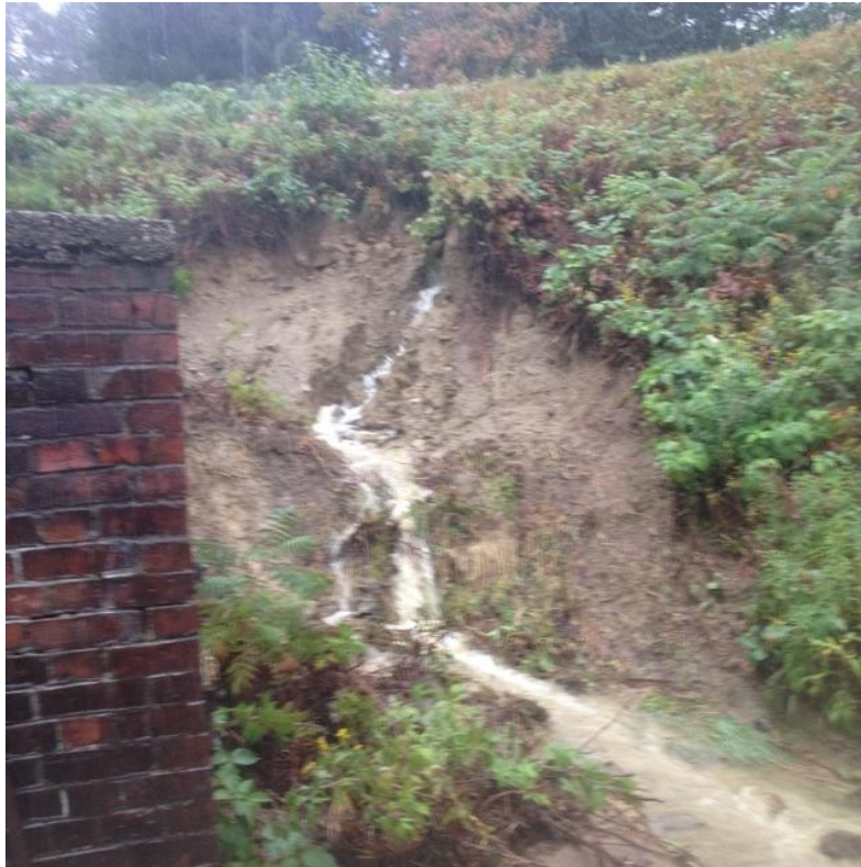
Battery B hillside collapse
