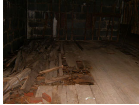
Powder magazine deterioration
